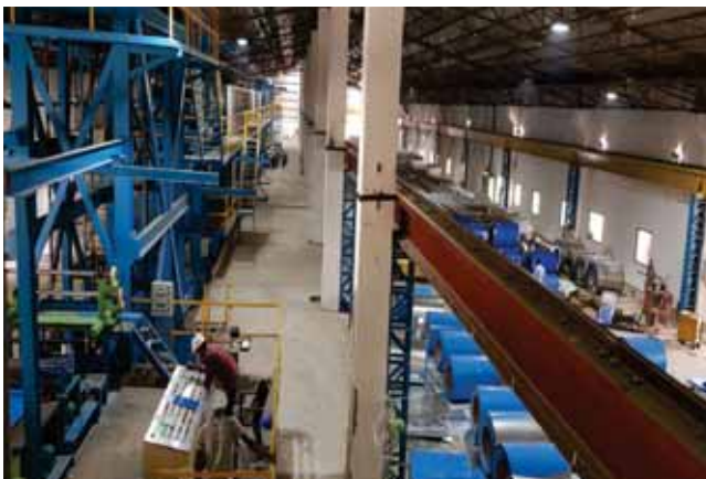
Colour coating Plant at Umbergaon, Gujarat
