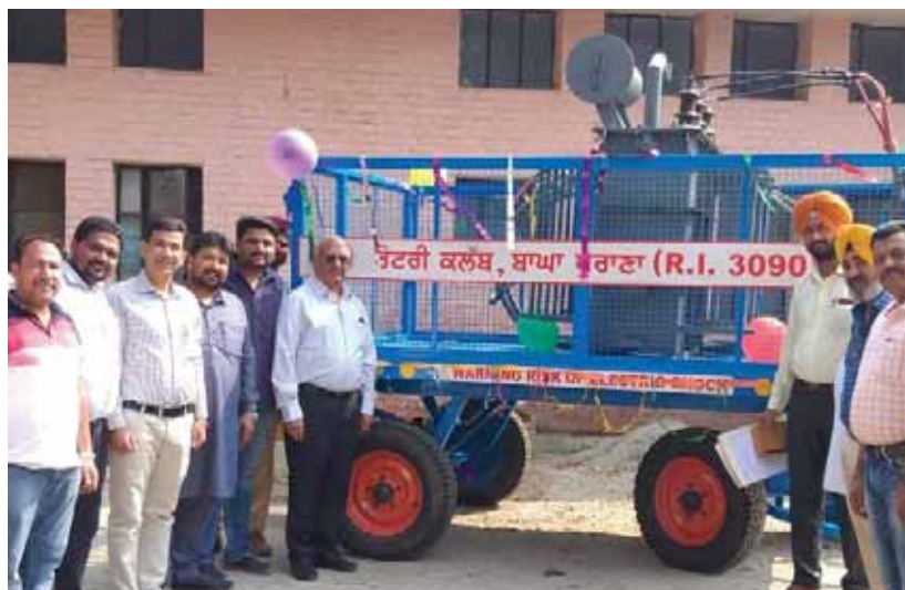
Rotarians with the Transformer on Wheels at a site.
