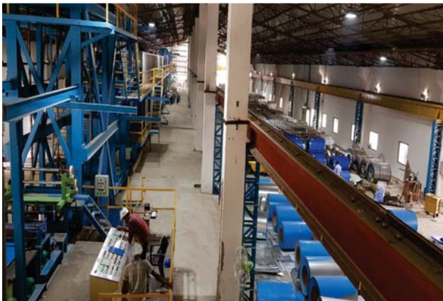
Colour coating Plant at Umbergaon, Gujarat
