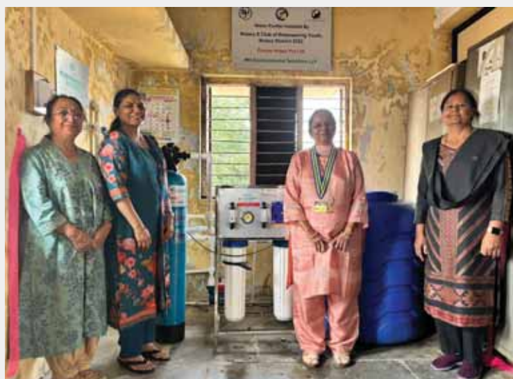
Water filter installed at the village school.
