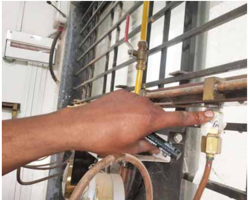
An ultrasonic machine being used to detect and plug leakage in an oxygen pipeline.
